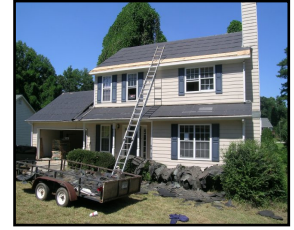
This is a house in the middle of one of our renovations: Fall 2008.
